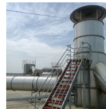
Organic Gas Exhaust Stack
